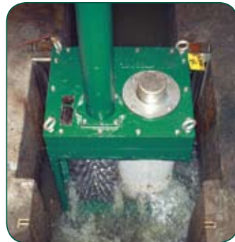
A model CMD replaced an old comminutor.
