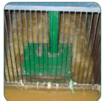
Channel Monster with overflow bar rack.
