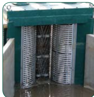
A model CDD6020-XDM2.5 installed in the inlet works.
