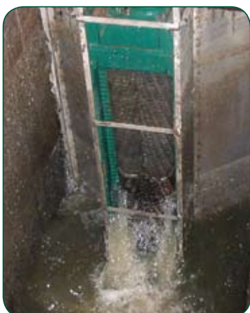
Muffin Monster in pump station
